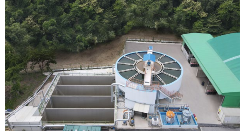
High-speed condensation precipitation tank
